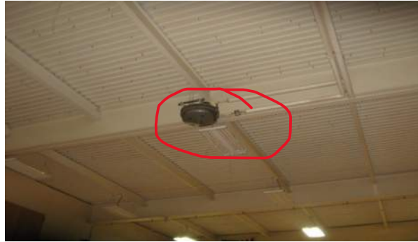
Gym Steam Unit Heater
