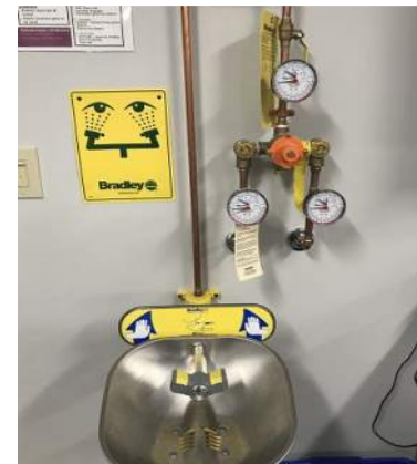
Example of new eyewash station
