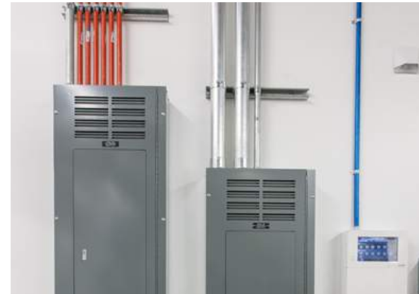
Example of new electrical panel
