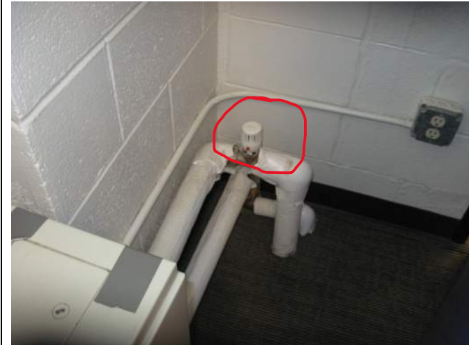
Boilers at North Mechanical Room
