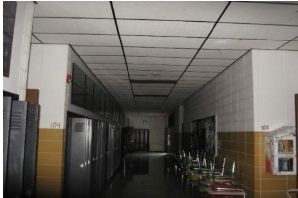
Corridor with no Emergency Lighting
