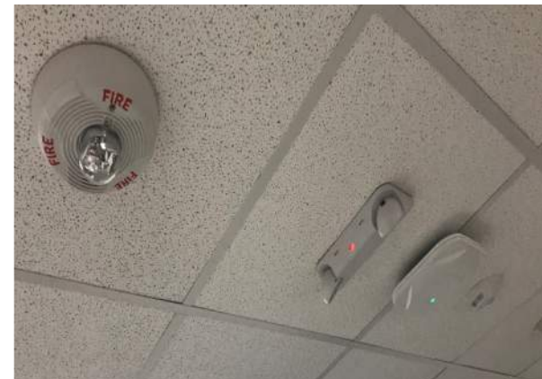
Example of new fire alarm system
