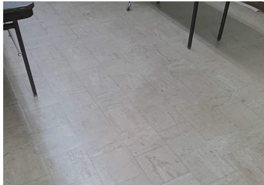
Existing asbestos containing floor tile
