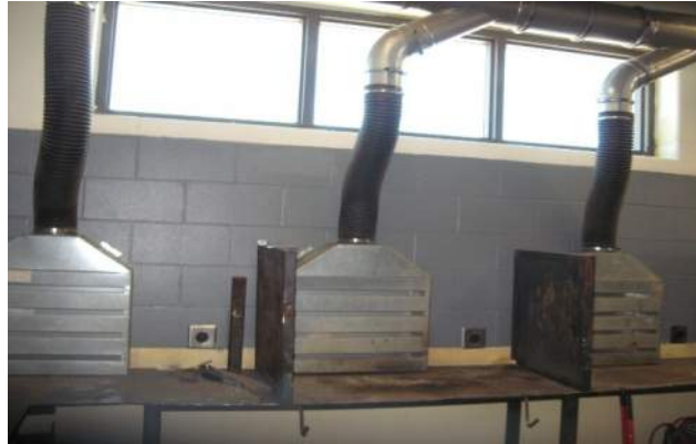
Needs Balancing Damper at Each Station
