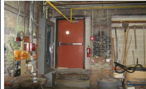
No E-stop Button at Door Entry/Exit
