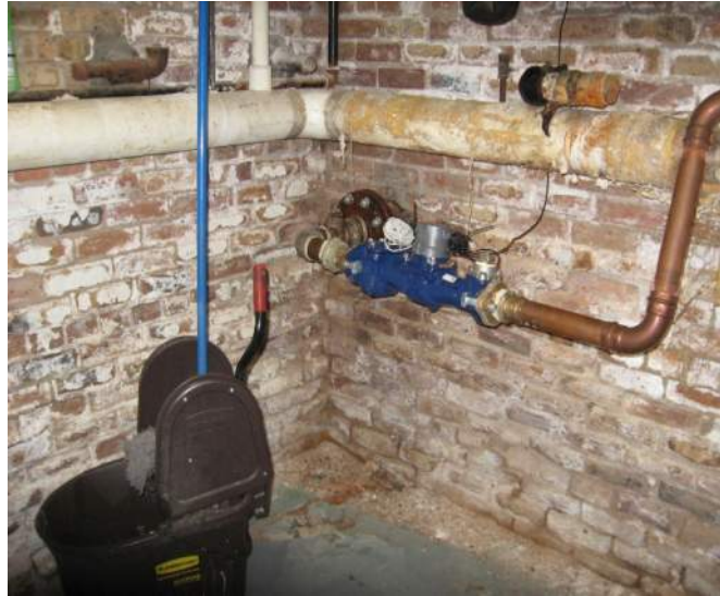
Missing Jumper on Water Meter
