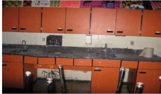
Receptacles Without Cover Plates
