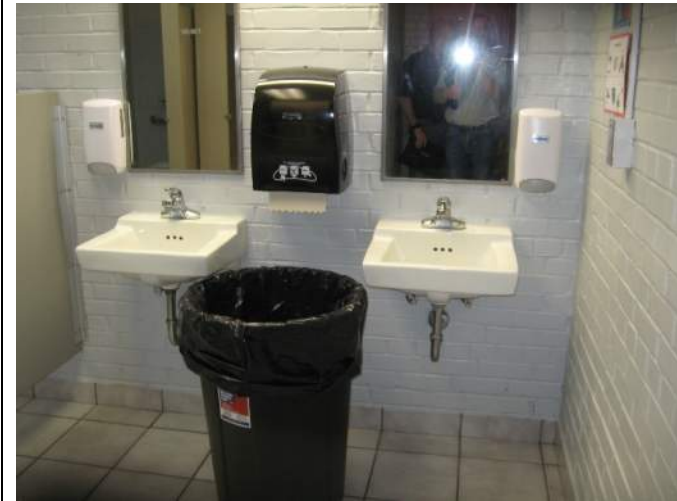
Sinks not to ADA Standards
