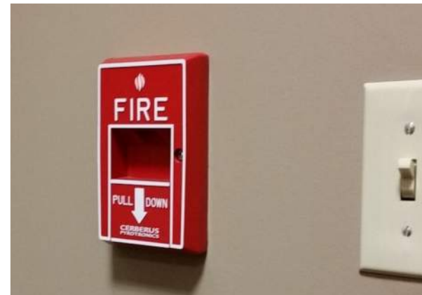
Example of new fire alarm system
