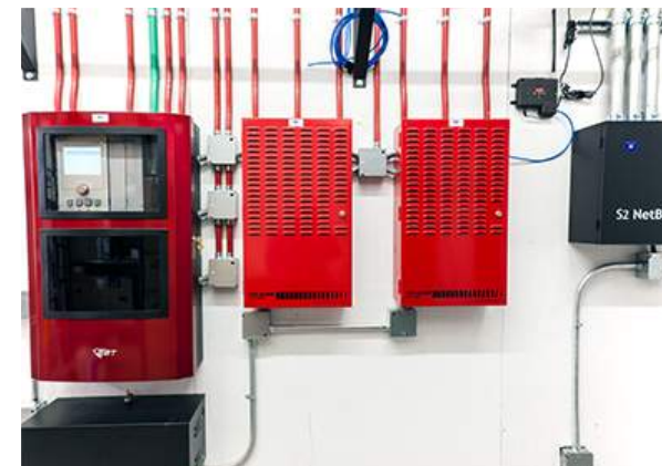
Example of new fire alarm system
