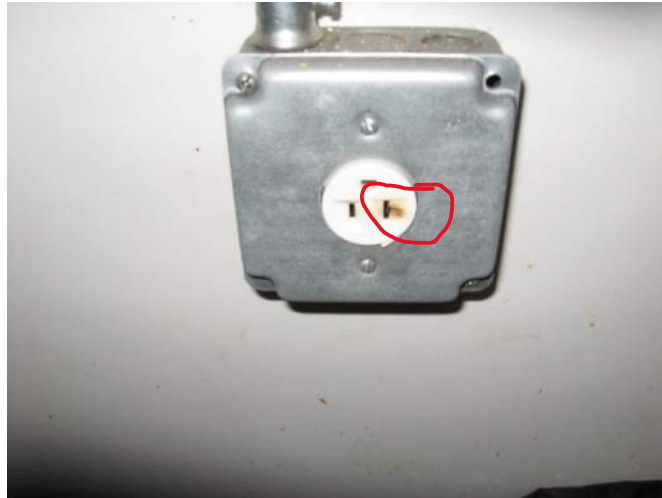
Receptacle Shows Signs of High Heat
