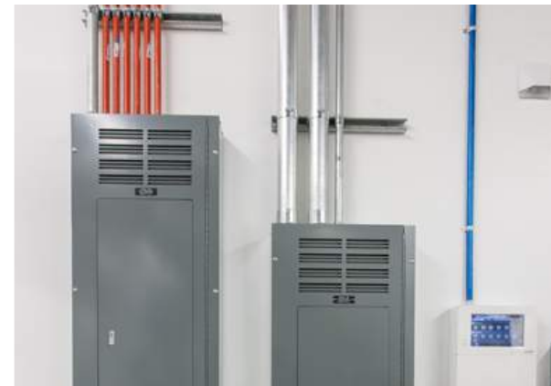
Example of new electrical panels
