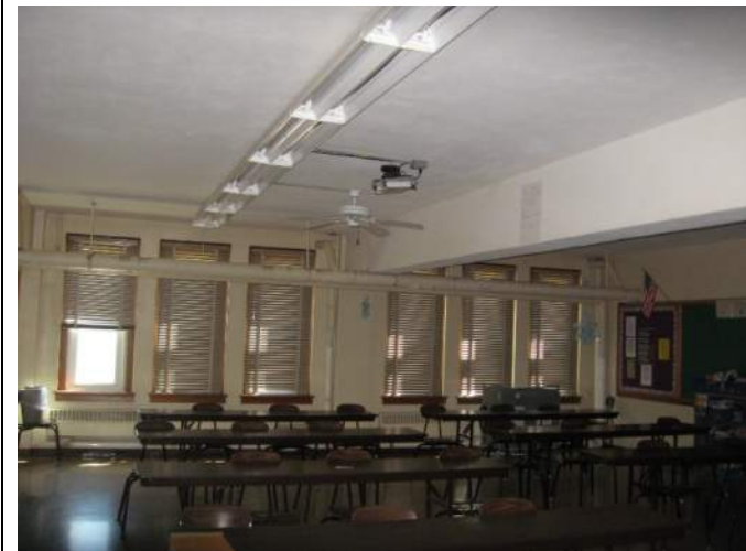
Room Showing no Smoke Detection
