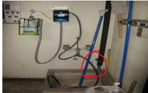
Faucet without a vacuum breaker
