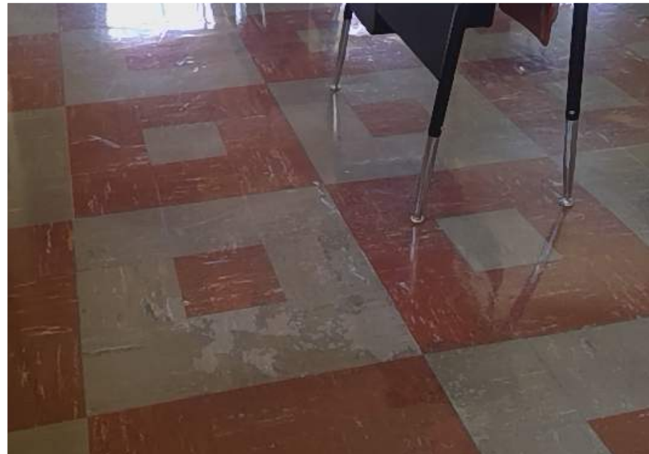
Existing asbestos containing floor tile
