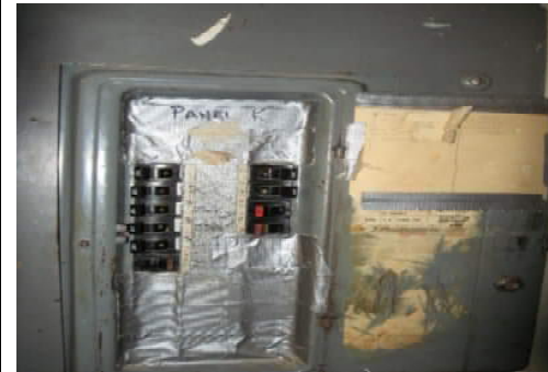
FPE Electrical Panel
