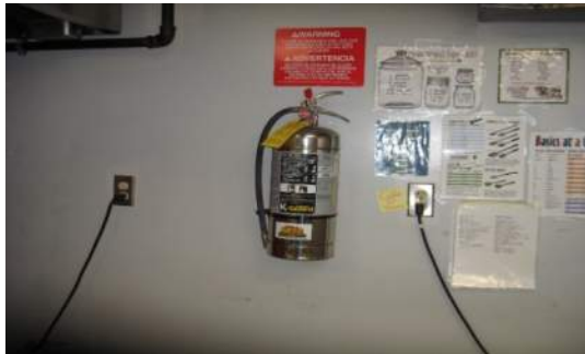
Non-GFCI Receptacles in Kitchen
