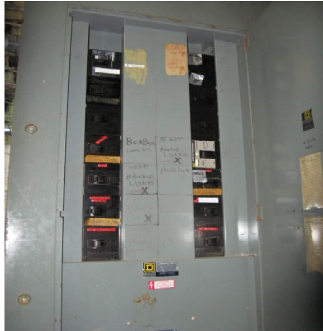
Electrical Distribution Panel
