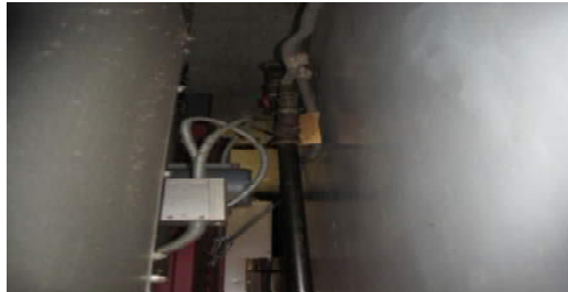
Electrical Equipment Under Kitchen Exhaust Hood
