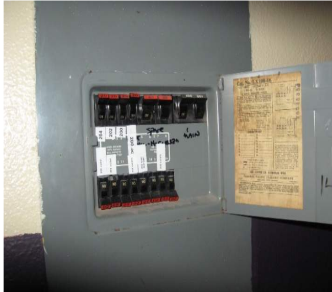
Federal Pacific Electrical Panel
