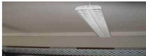
Old Fluorescent Light Fixture
