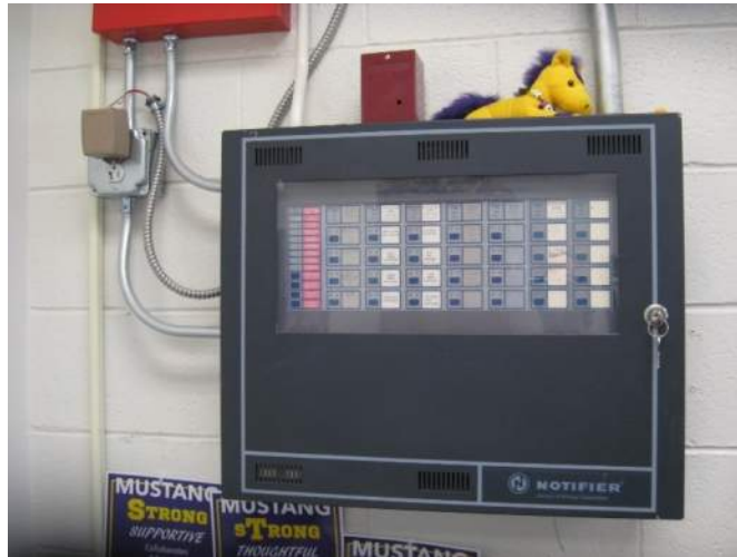
Fire Alarm Panel
